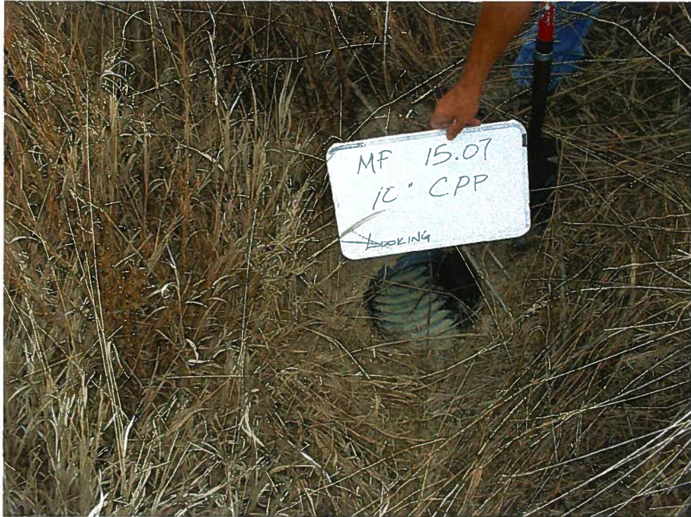
Mile Post 15.07 10" CPP North End
